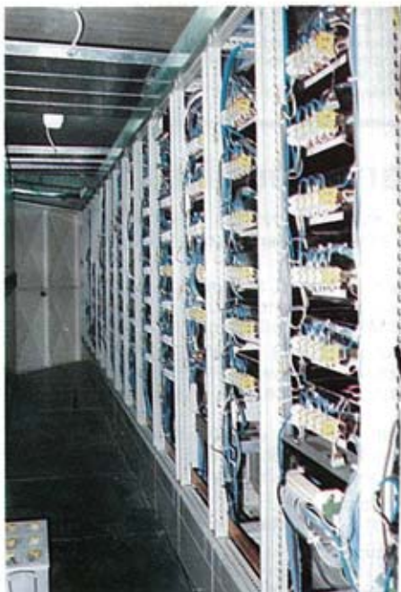
The Winter disco central dimmer room.
